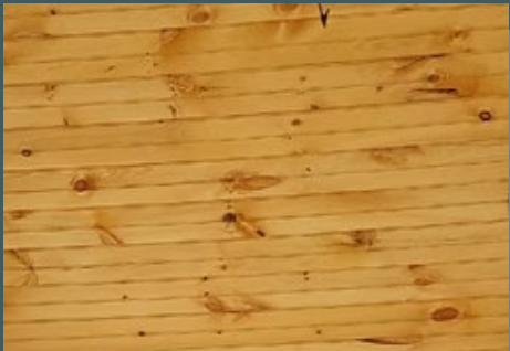
*stained covered rafters
